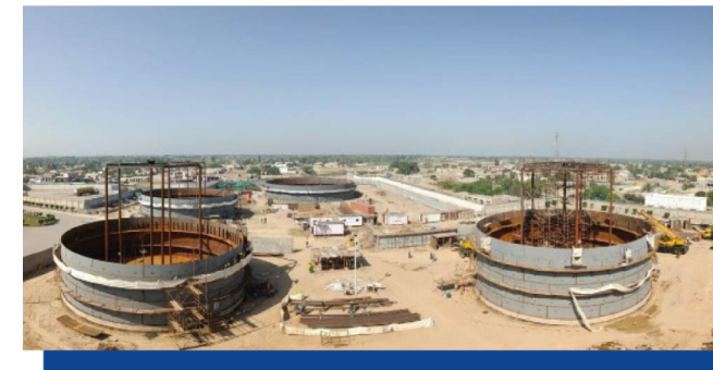
Construction of 4 tanks of both HSD & PMG with the capacity of 22,000 MT & 24,000 MT respectively
