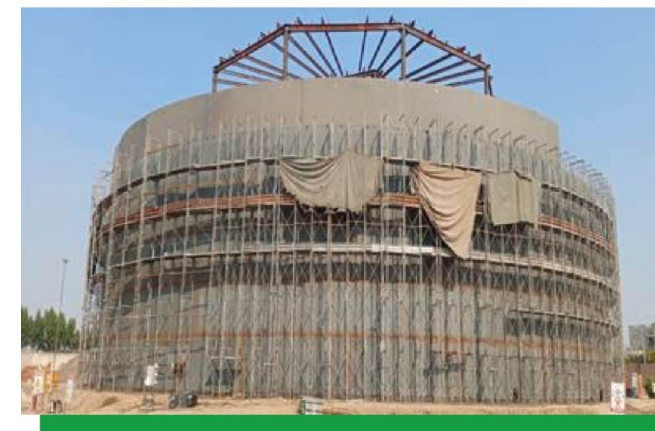
Construction of PMG Tank of Capacity 20000 MT is in progress at Faisalabad Depot
