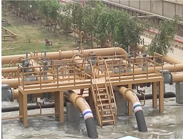
Initiation of gasoline movement through white oil pipeline
