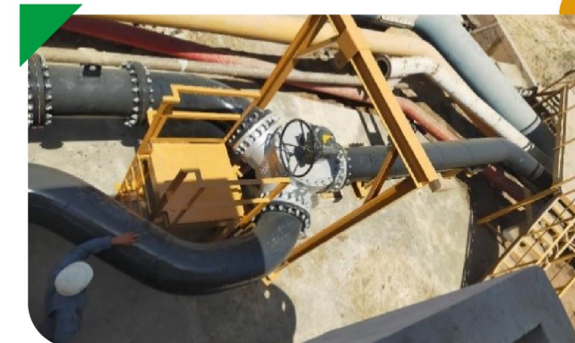
Commissioning of three-way valve system on the 20" Diameter Tank discharge line (TDL) at Keamari, Karachi
