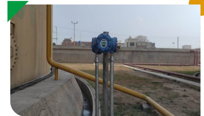
Installation of advanced radar gauging system with smart wireless technology on storage tanks at Keamari Terminal B (KTB), Faisalabad, Mehmoodkot and Sihala.
