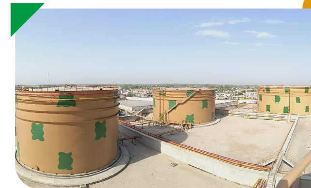
Construction of 7 new tanks at Faisalabad (1 new tank with a total capacity of 20 KMT), Faqirabad (2 new tanks) and Mehmoodkot (4 new tanks with a total capacity of 46 KMT)
