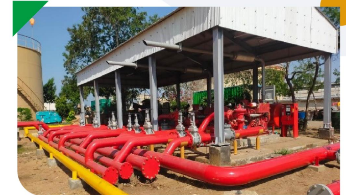
Completion of construction activities for firefighting upgradation projects at 07 locations: Keamari Terminals A & C, Daulatpur, Tarujabba, Habibabad, Faisalabad and Faqirabad depots
